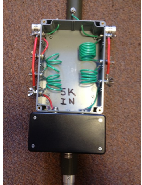
Figure 1. Interior of the coil box with cover removed, showing coil arrangement after modification.
